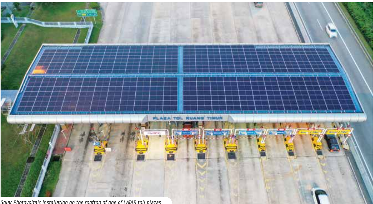
Solar Photovoltaic installation on the rooftop of one of LATAR toll plazas
