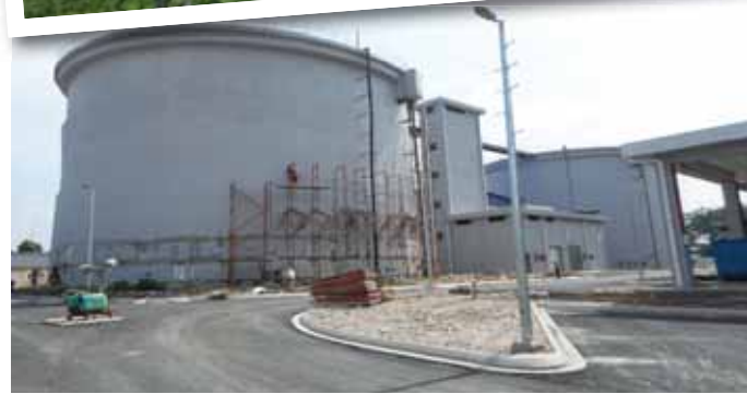
Bunus Regional Sewage Treatment Plant, Kuala Lumpur
