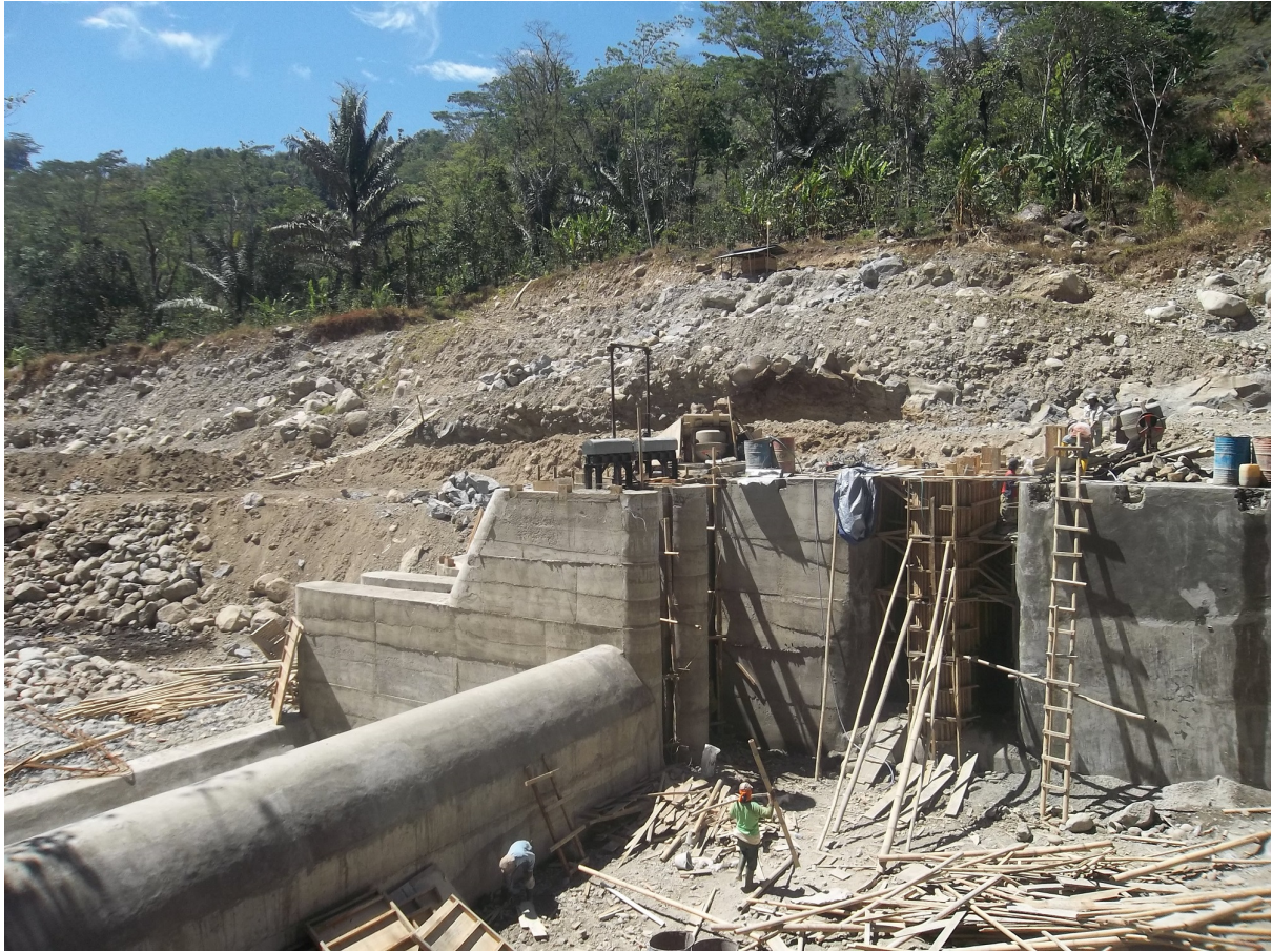
Mini Hydro Power Plant in Bantaeng Sulawesi, Indonesia
