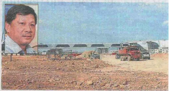
The unfinished taxiway of KLIA2. Tee (inset) says there have been many last-minute requests and additional changes made by stakeholders of the new airport.
