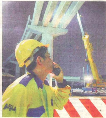
Team effort: It took a crew of 100 men and three engineers to put in place the final beam.
