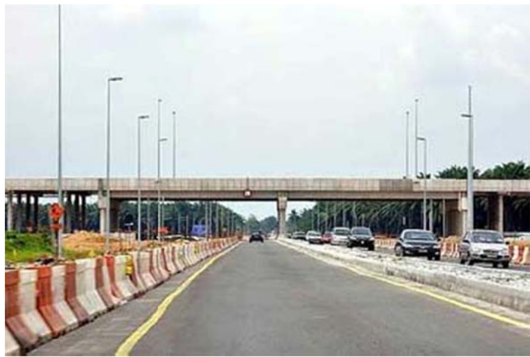
Near completion: The Latar Expressway stretches over Jalan Bukit Besar Rotan near Ijok.
