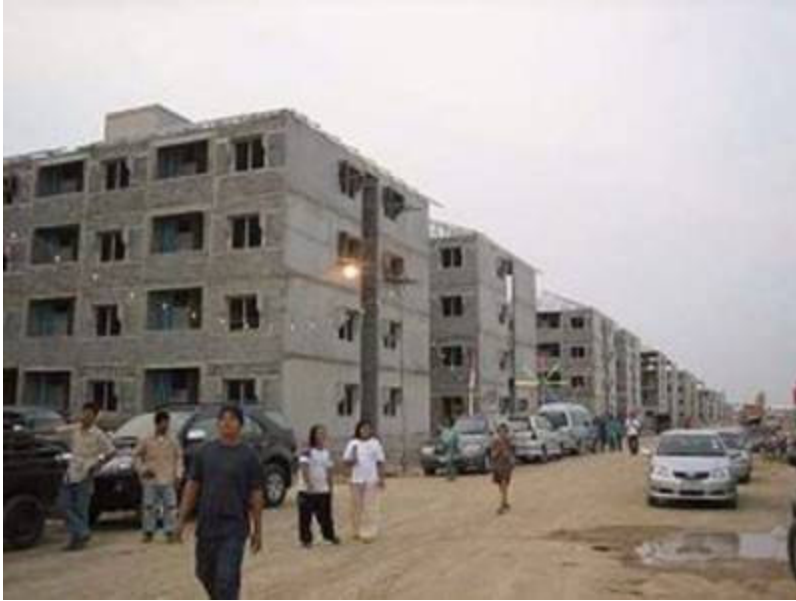
Construction of the four--storey apartments in Bang Pu province by Bina Puri Thailand Ltd.
